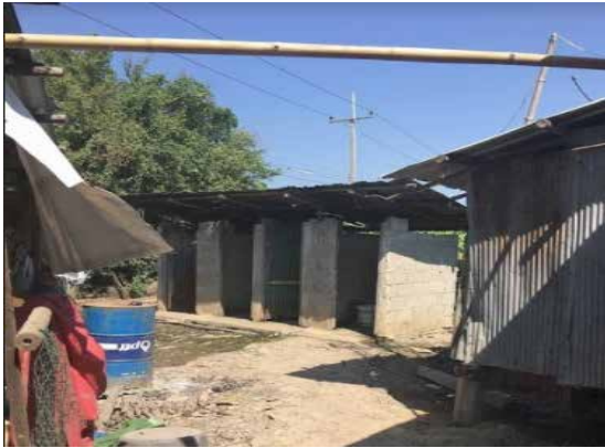
Toilets before renovation
